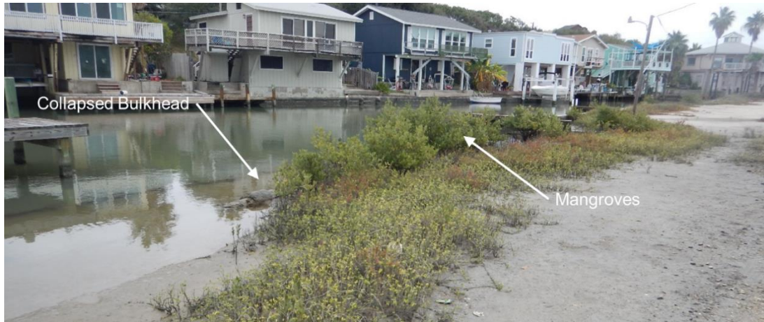
Figure 23. Exposed shoreline along South Sandpiper Street.
